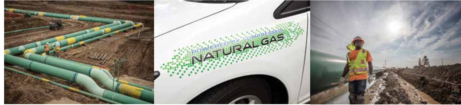
The newly completed Nexus pipeline is delivering natural gas across northern Ohio.
